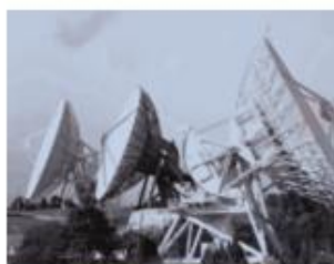
通信设备 Communication Equipment
